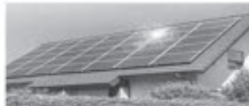
ON GRID & OFF GRID SOLAR PLANT
